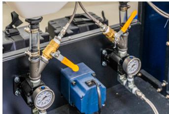
2 BALL VALVES TO FLUSH PUMP LINES
